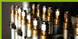
Compressed air distribution in the ÖKOBIT pump container
